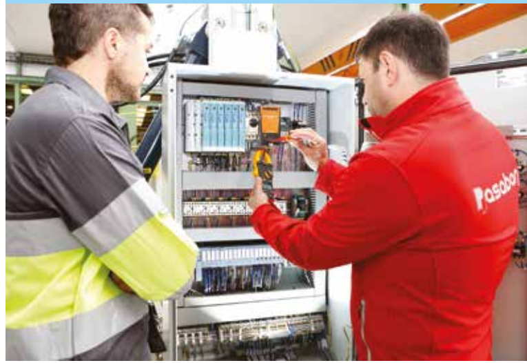
Image 4: Electric cabinets for automation control.
