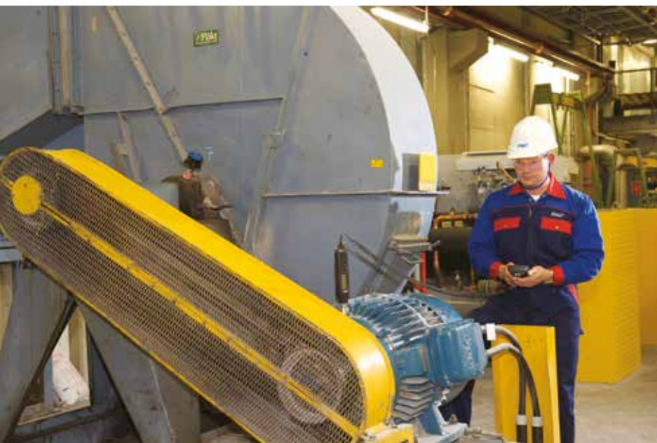
Image 6: Fan at UPM Schongau.
