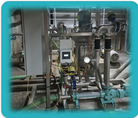
Figure 2: Jet Wing Liquid Filter in the basement of a folding-boxboard machine
