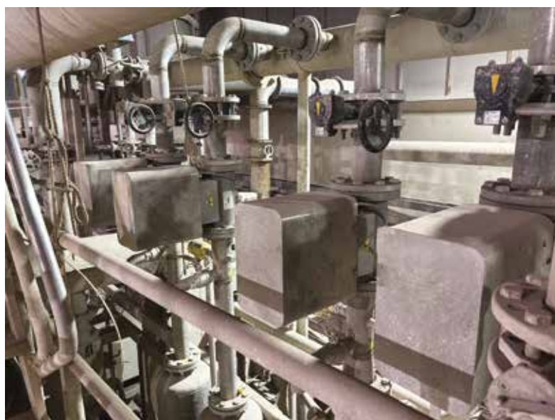
Image 4: OraStream valves after installation.
