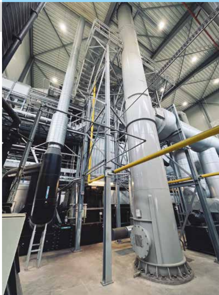
Figure 5: Interior of the CPH plant.
