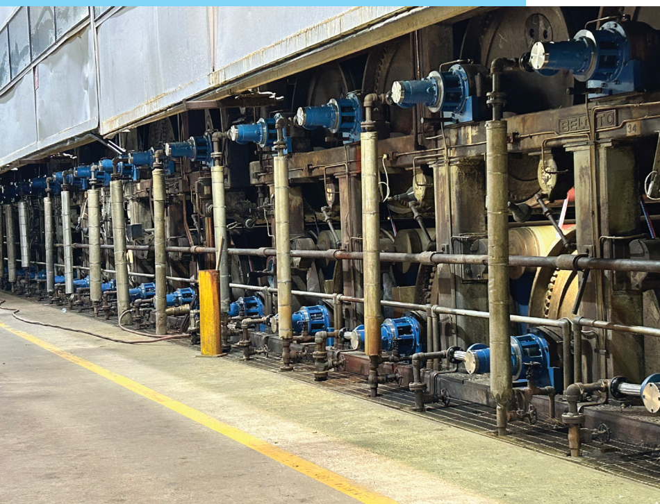
Figure 1: Dryer section featuring newly installed condensate outlet unions.
