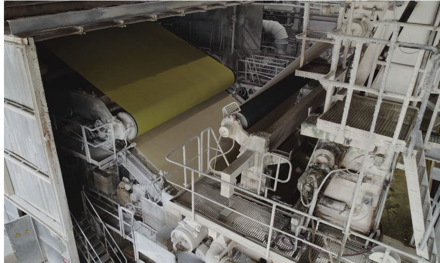
Figure 3: (Above) Forming and press section with Wefapress dewatering elements.
