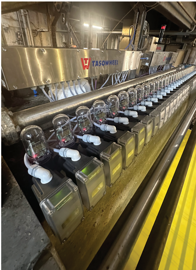
Figure 2: DigiForte actuators installed side by side.
