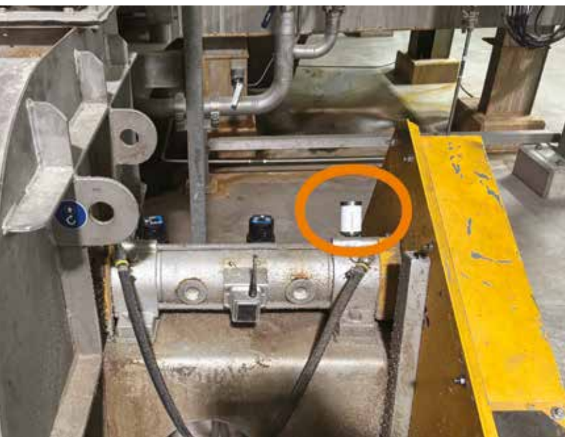
Figure 2: Endiio V2 Sensor installed at a ventilator's bearing.
