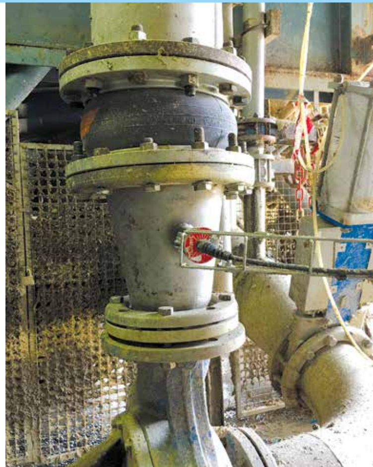
Figure 1: BTG Optical consistency transmitter TCR-2511 installed at the outlet pulper
