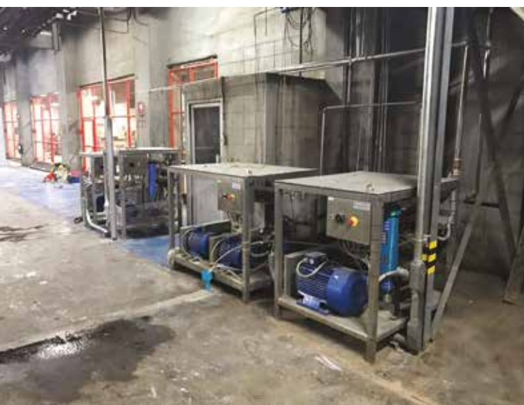
Figure 3: Multiple ProJet pump stations for Forming Fabric, Press Felt and Dryer Fabric Cleaners.
