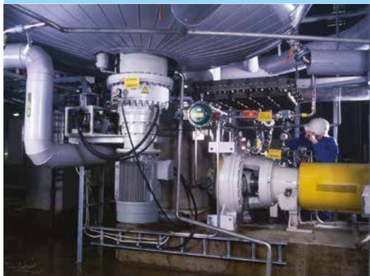
Figure 11: MC tower discharge pumping system.
