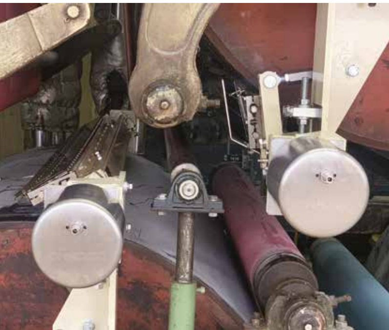
Figure 4: OraFlex drying section (Left).
