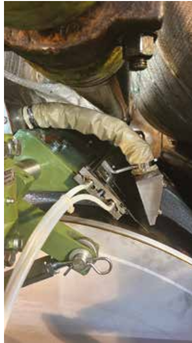
Figure 7: Dust removal system.
