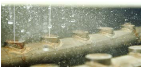
Fig. 2: Functioning and clogged nozzles
