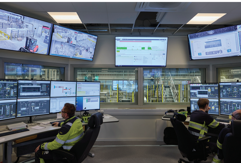
Figure 11: Inside control room.
