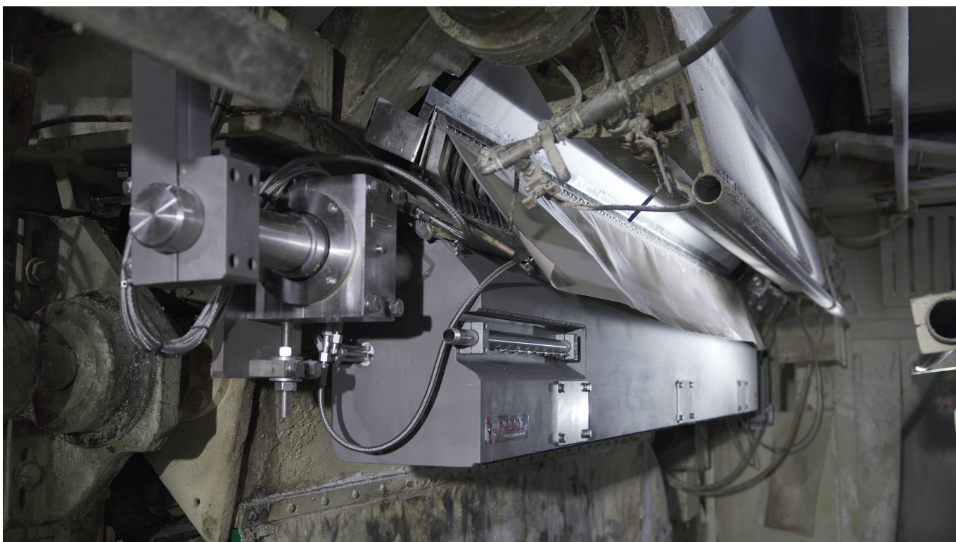
Figure 2: Overview of OraCrepe Next installation.
