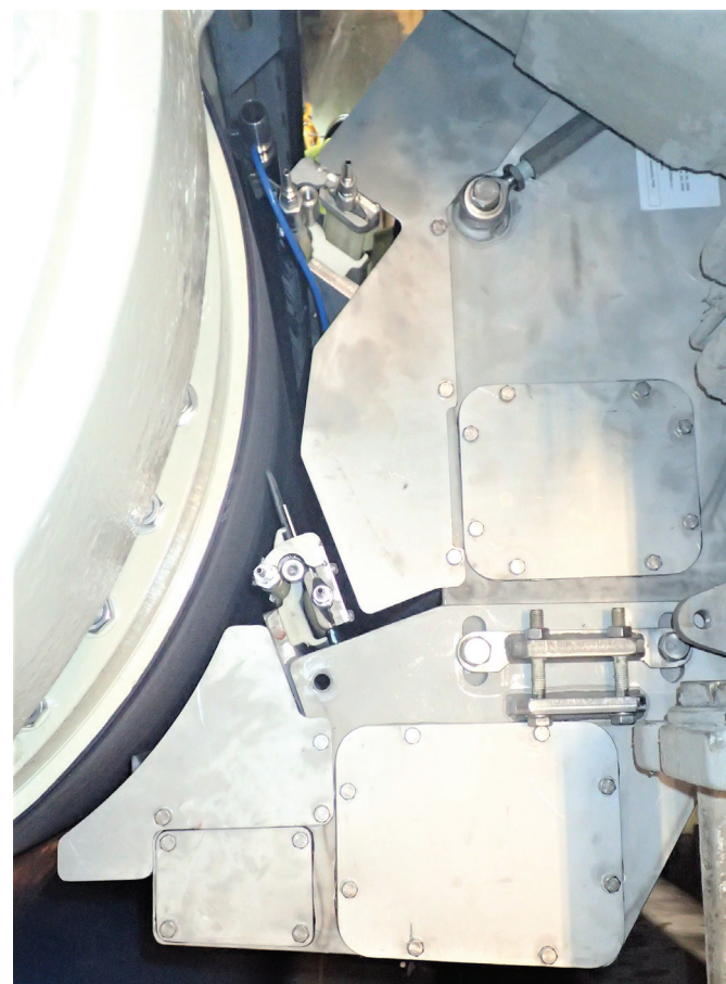
Figure 5: A well-designed and operated dewatering and doctoring system is one of the key issues to a well-performing and energy-efficient machine.
