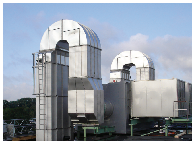
Figure 6: Heat recovery, as an important part of the RunEco solution, cuts down papermaking energy costs radically because the system reuses heat to replace primary energy sources
