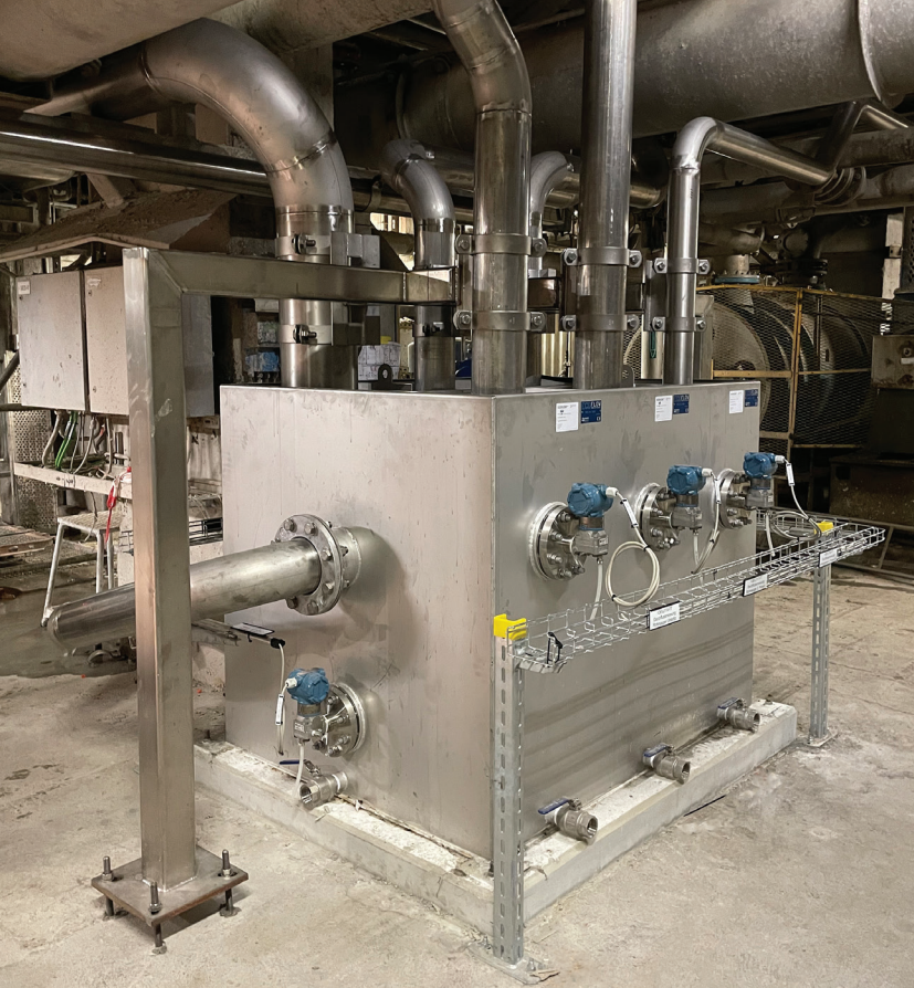
Figure 4: EcoFlow is the only reliable and accurate online dewatering measurement system for water that contains lot of air. When you measure the water flow accurately, you can adjust the vacuum optimally and reach high energy efficiency.
