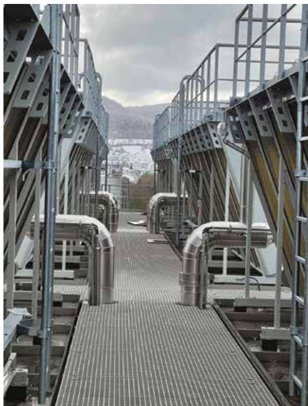
Figure 5: Drycoolers “Drycoolers to provide freecooling up to 14 °C Outside temperature”.
