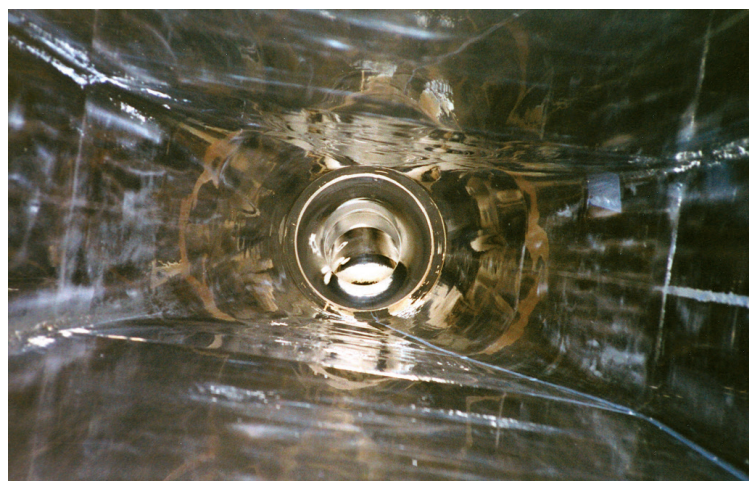
Figure 7: Same headbox after successful cleaning, barium sulphate scale removed.
