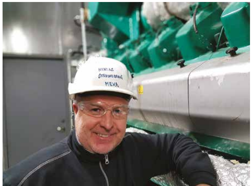
Figure 4: Meva Energy's CHP demo plant with Cummins Genset and capacity of producing 1,2MWe and 2,4MWth
