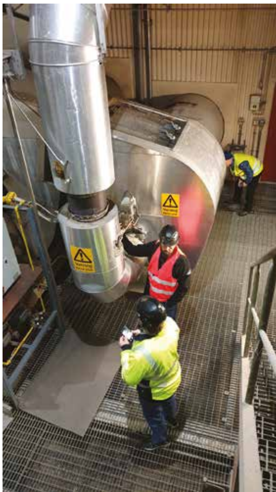
Figure 1: Example of combustion chambers at a tissue mill, generating heat for the drying hoods.
