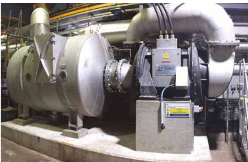
Figure 1: Vacuum system audit is a tool to document and benchmark the vacuum system and sheet dewatering effectiveness, to highlight problem areas and illustrate options to reduce operational cost associated with the vacuum system.
