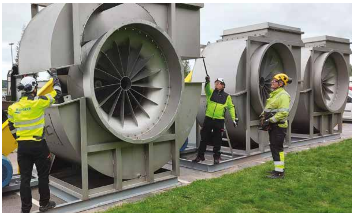
Figure 7: Hood exhaust fan assembly on site. Modifications to existing machine hall ventilation systems can be done by installing additional ventilation units, both supply and exhaust air units, locating them in positions where they give the best benefit.
