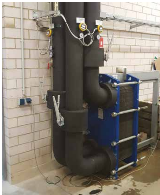
Figure 6: Plate heat exchanger for the riverwater
