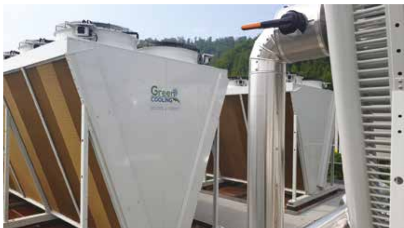
Figure 1: 3MW of free-cooling power with dry-coolers.
