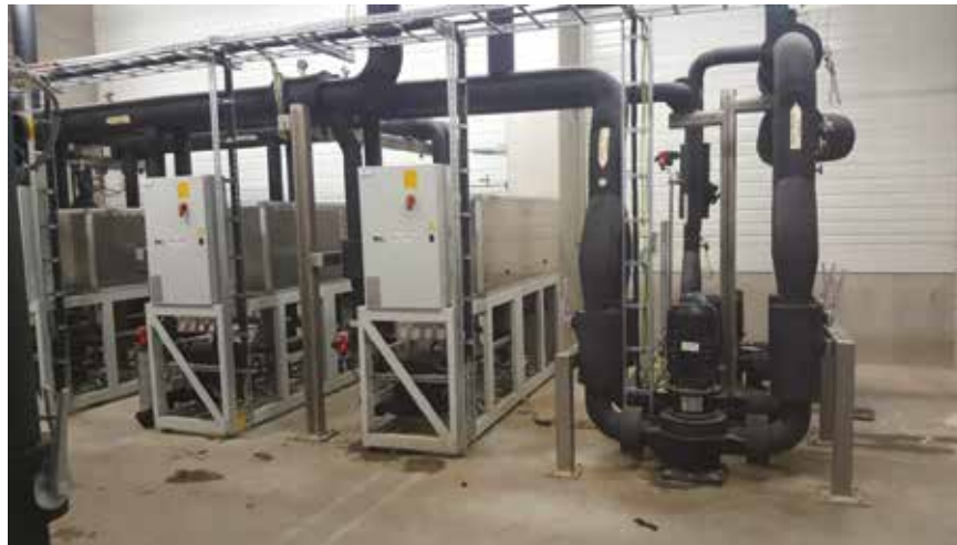
Figure 2: Chillers for redundancy and for warmer times of the year.
